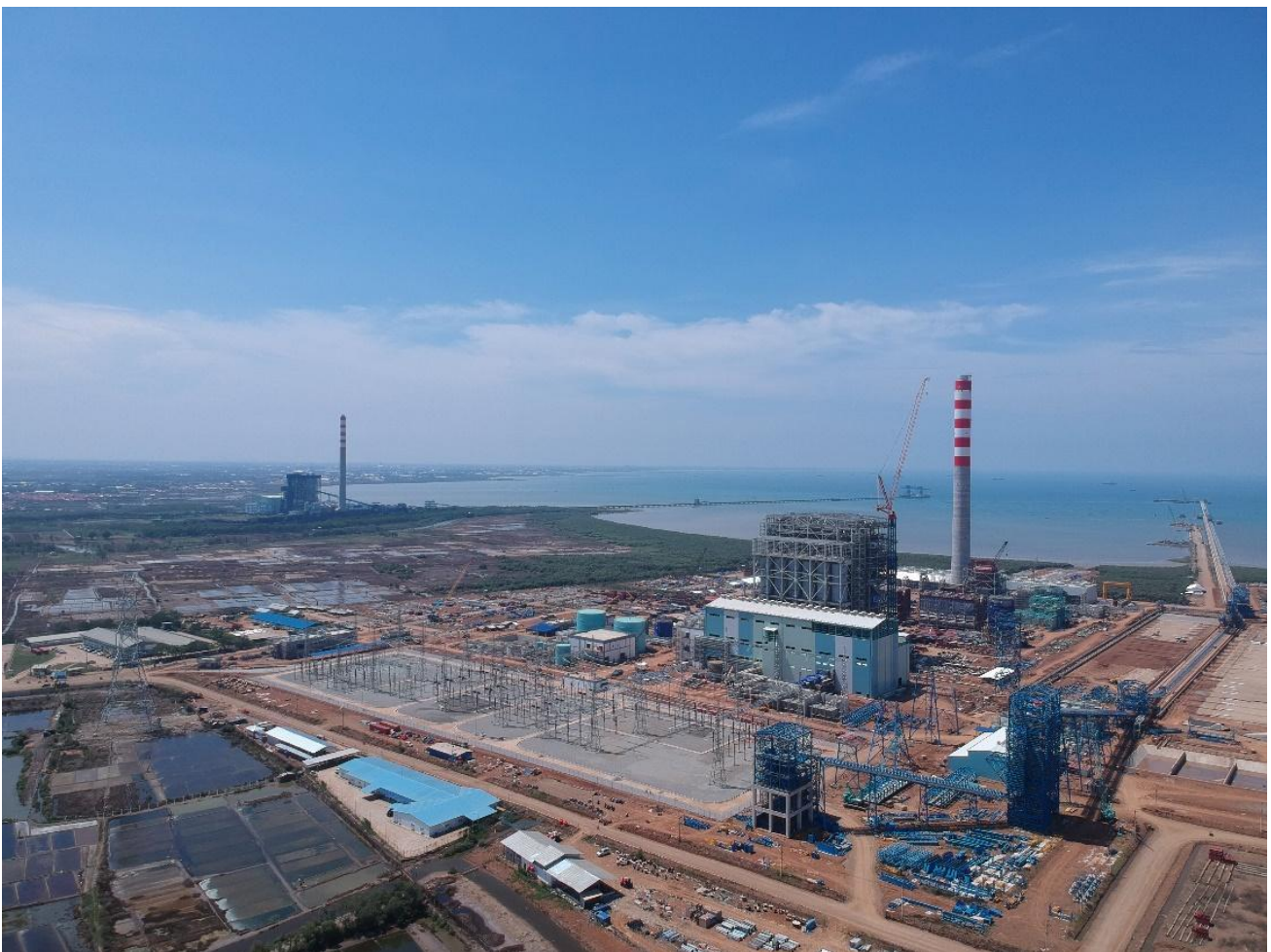
Photo: Cirebon Coal Fired Power Plant Unit 1 (in distance) and Unit 2 (foreground, under construction) (WALHI (Indonesian Forum for the Environment) West Java, Oct. 2020)
